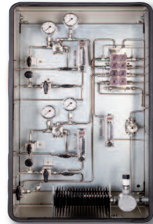
Custom Sample Conditioning System
